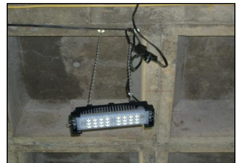
Image2: LED Temporary Light
